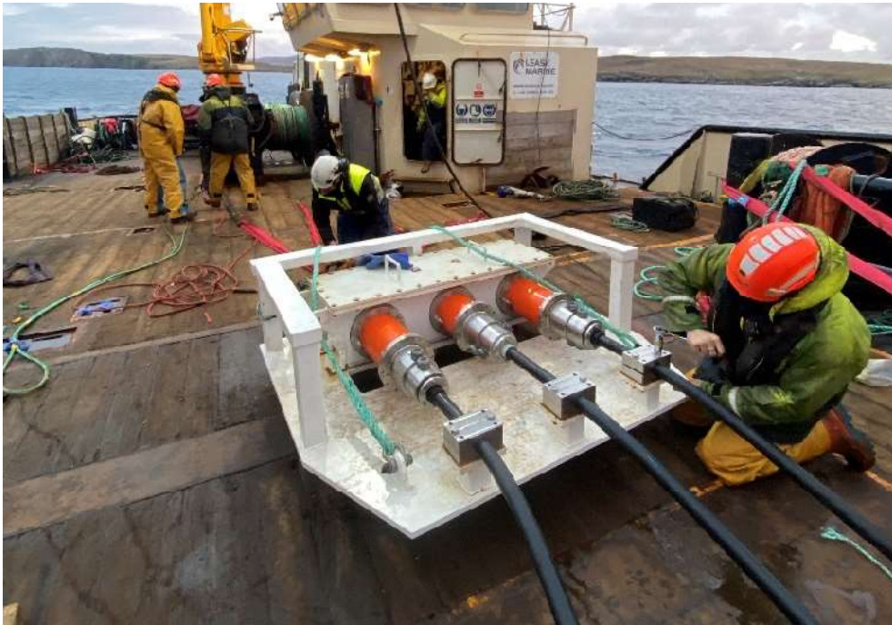
Figure 9-5: T5/T6 subsea cable hub on deck prior to installation
