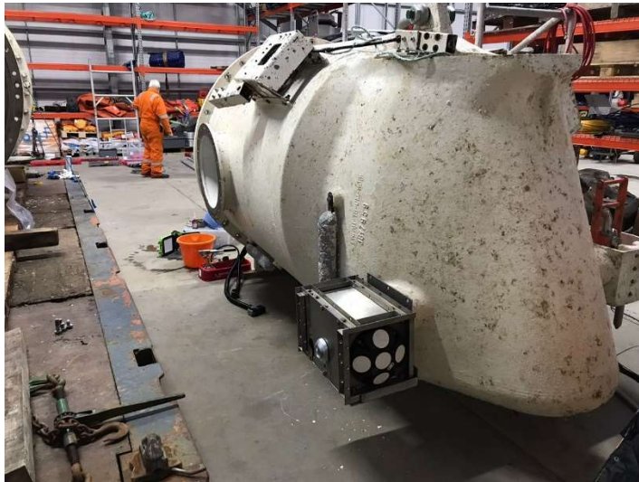
Figure 8-7: Nacelle-mounted ADCP installed on turbine T4
